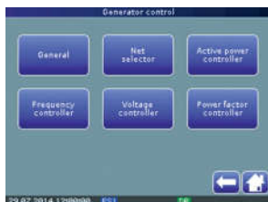
SYMAP® GC: Generator Control Functions
